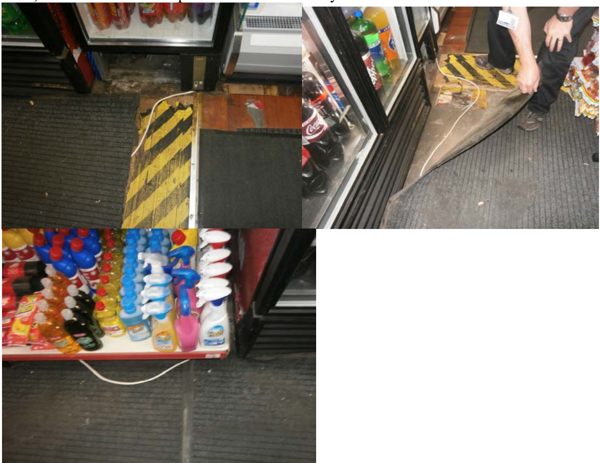
2) Cable run under carpets and across walkways.
