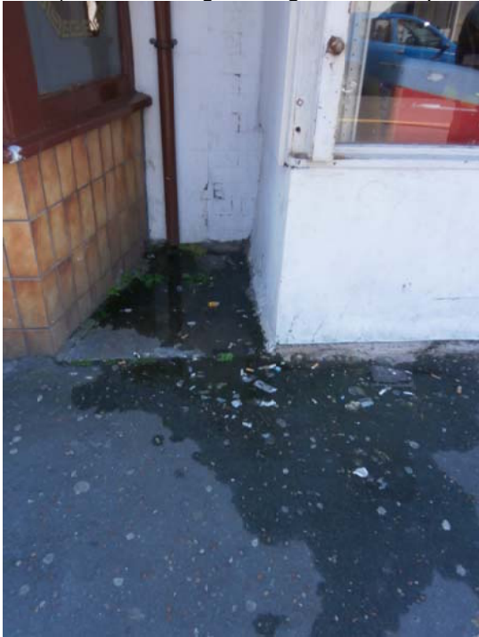
1) Overflowing drainage to front of premise
